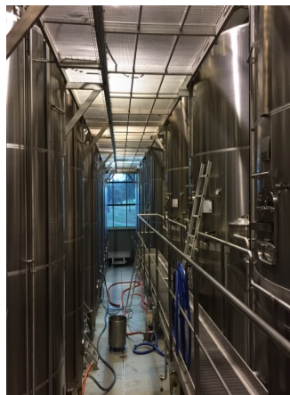
Stainless steel tanks
